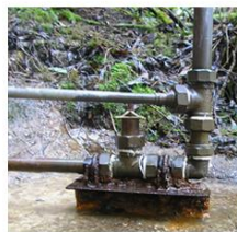
Delivery Pipe - pipe from the ram pump to a collection tank
