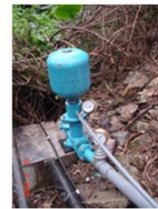
Pressure Vessel - serves as a buffer and catch up the over pressure
